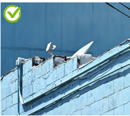
Locate satellite dishes and mechanical equipment out of public view. This dish is mounted on the rear of the building behind the parapet.
