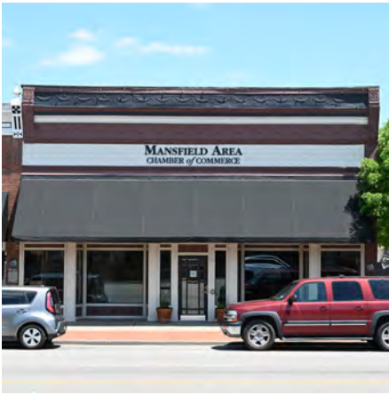
Skylights should not project above the parapet. The skylight on this building is hidden by the front parapet.
