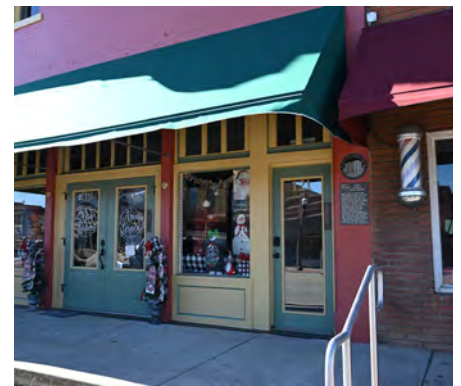
The color of awnings should be compatible with the exterior color of the building. This green awning fits with the building's color scheme.
