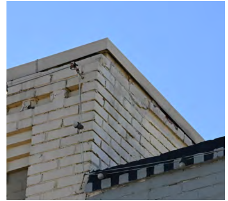
Applying paint or stucco to masonry can seal in moisture and cause damage to the material. The brick in this wall was damaged after water was trapped between the paint and brick.
