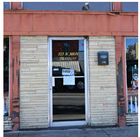
Use a door associated with the building style. This entrance with a Mid-Century door is not appropriate for the building style.
