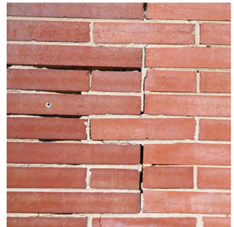
Repoint mortar joints where deterioration is evident, as seen on this section of wall.
