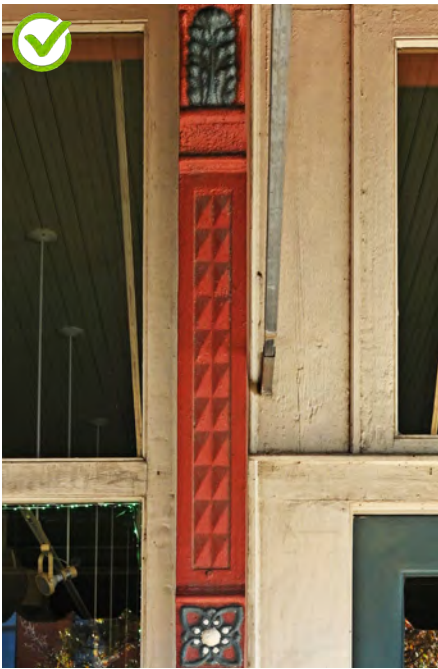
Maintain protective coatings like paint on exposed metals. The paint scheme on this column not only preserves a significant architectural feature of the building, but also highlights the column's decorative details.
