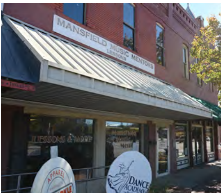
Do not cover or obscure significant architectural features. This awning covers the transom windows.
