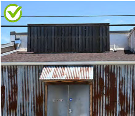
Screen equipment from public view. The roof-top HVAC units on this building are set back from the rear wall and screened by a board-on-board enclosure.
