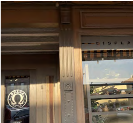
Where an architectural detail is missing or damaged beyond repair, alternate materials may be considered. This is a replica of a cast iron column that was removed from the building earlier.
