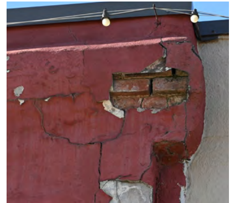
Remove coatings like paint and stucco from masonry surfaces if it can be done without damaging the masonry. It may be possible to remove the stucco from this parapet, but testing is necessary.
