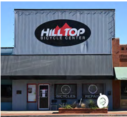
Consider removing any covering which obscures the original materials from view. This slipcover hides the upper story window openings and historic masonry.
