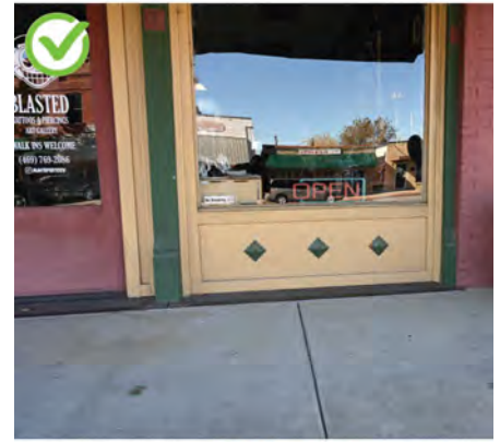
The top of a bulkhead should generally align with the bottom panel of a traditional door. The bulkhead above is close to the same height as the top of the bottom panel on the door.
