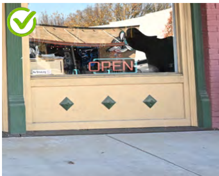
The wood bulkhead and the cast iron threshold seen here are important features of this historic storefront.
