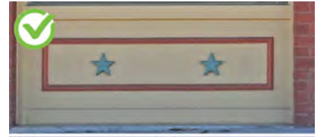
Wood is an appropriate material for replacement bulkheads on vernacular storefronts. This replacement wood bulkhead is designed in a traditional style that complements the storefront.
