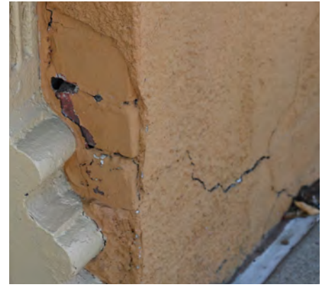
When this stucco deteriorated, the exposed brick was damaged by water. A maintenance plan can ensure that regular inspections and appropriate maintenance are carried out in a timely manner before major repairs are needed later.
