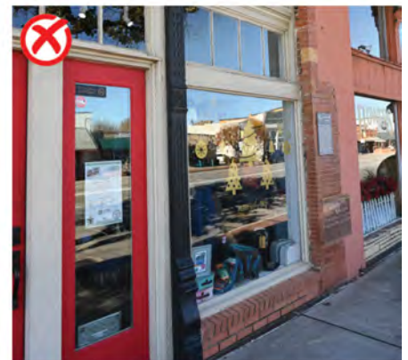
This replacement bulkhead is shorter than the original. It changed the scale of the original historic storefront. Compare to the original storefront in the photograph above.
