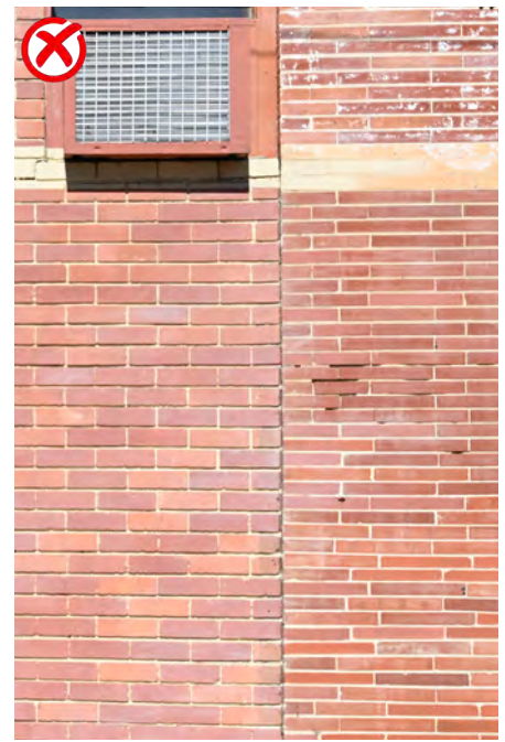
New brick should match the original in size, color, material composition and mortar. The brick on the right side of this photograph is the original brick. The modern brick on the left was used to repair a large section of wall. The new brick is not the same size or material composition of the original and is not an appropriate material for this building.
