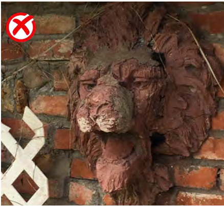
Do not remove architectural features that are in good shape or can be repaired. This lion's head ornamented a historic bank but was broken into pieces when it was removed from the building. The pieces were patched together with Portland cement, causing permanent damage to this feature.
