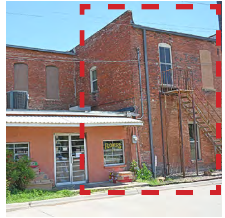
Preserve an older addition that has achieved historic significance in its own right. The 1910 addition to the Masonic Lodge Building has become a historic structure in itself and should be preserved. The newer addition to the left could be considered for removal.
