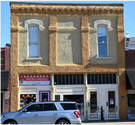
Stucco covers the masonry walls of this 1892 building. Removing the stucco must be done with care to avoid damaging the historic brick.
