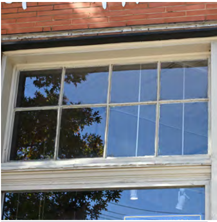
Wood was historically used for trim and ornamental details. Repaint or treat wood elements when the surface shows signs of deterioration.
