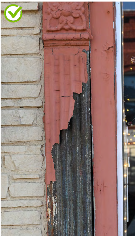
Remove rust from metal features, caulk and repaint as necessary.
