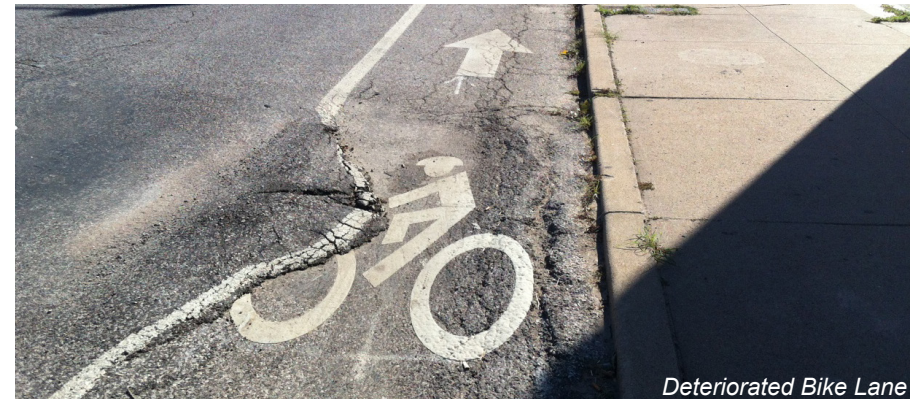
Deteriorated Bike Lane
