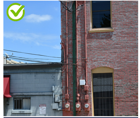
Locate utility lines and junction boxes on secondary and tertiary facades, and group them where possible. These electric meters are grouped together on the rear wall of this building.
