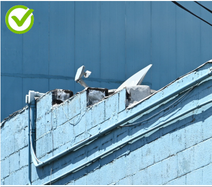
Locate satellite dishes and mechanical equipment out of public view. This dish is mounted on the rear of the building behind the parapet.
