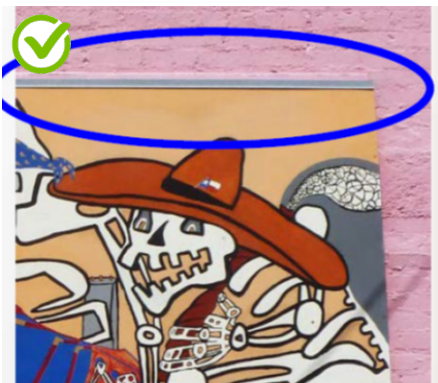
Prevent water from getting trapped behind the mural. The cap on this mural directs water away from the wall.
