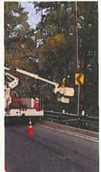
Electric & Existing Pole
